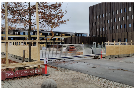
DTU Campus Service is erecting fences around the construction site for Building 313. In the background is Building 310. Photo: DTU
